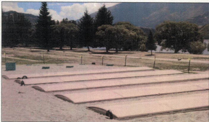
This array of AX-Max units provides wastewater treatment for a large resort and camping area in New Zealand.
